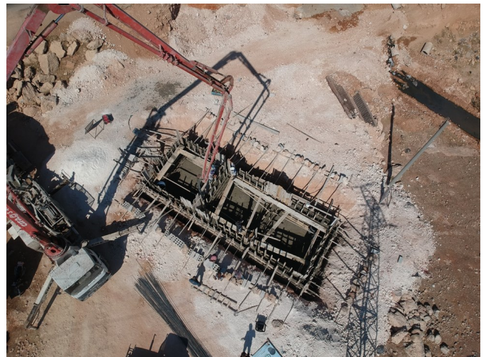
Construction works of multi-chamber septic tank in an IDP site in Idlib – Northwest Syria © IOM 2020, through WATAN Foundation.
